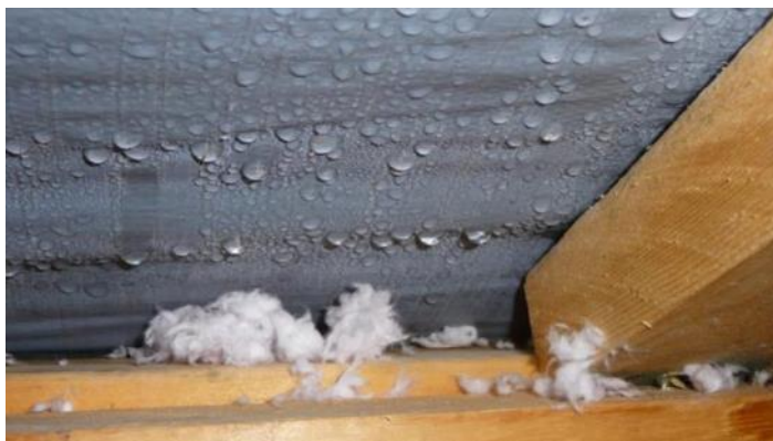
Figure 1 – Condensation in roof space (Photo retrieved from Agassiz Roofing, agassizroofing.com)
