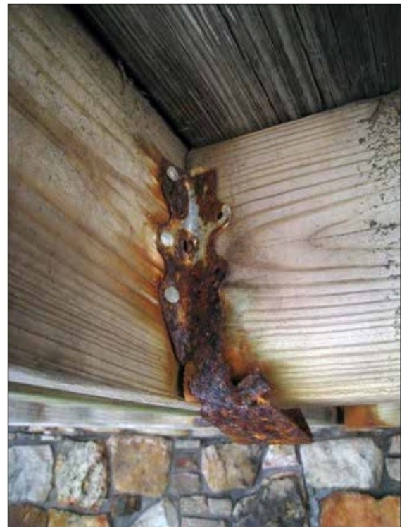
Photo 2: An ordinary galvanised joist hanger in an exposed environment
