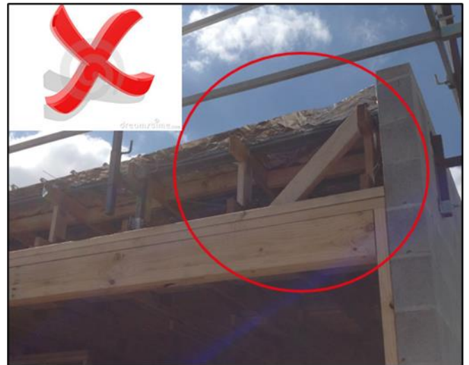
Photo 1 – Non-complying vertical end bracing
