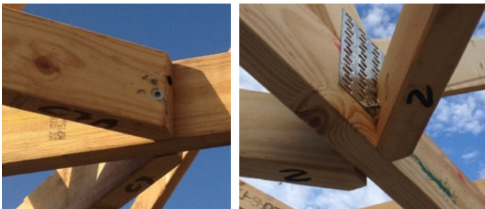
Figure 4: Screws in use with inadequate edge distance or embedment
